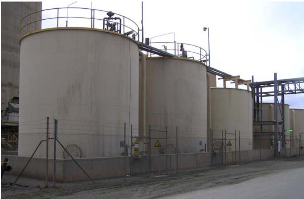
Figure 1.3 Elution Solution Storage tanks at Fimiston (F66 Goldroom)
