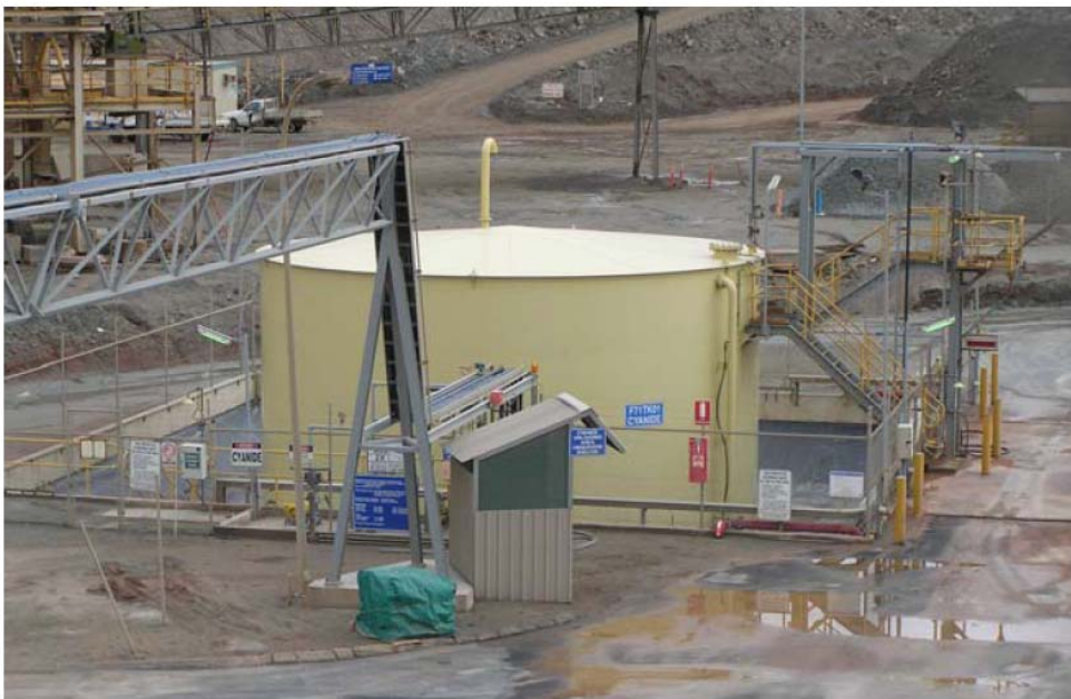
Figure 1.1 Cyanide Storage Tank at Fimiston (F71TK01)
