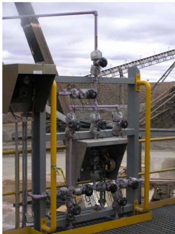
Figure 1.2 Cyanide Dosing Manifold at Fimiston (CIL1)
