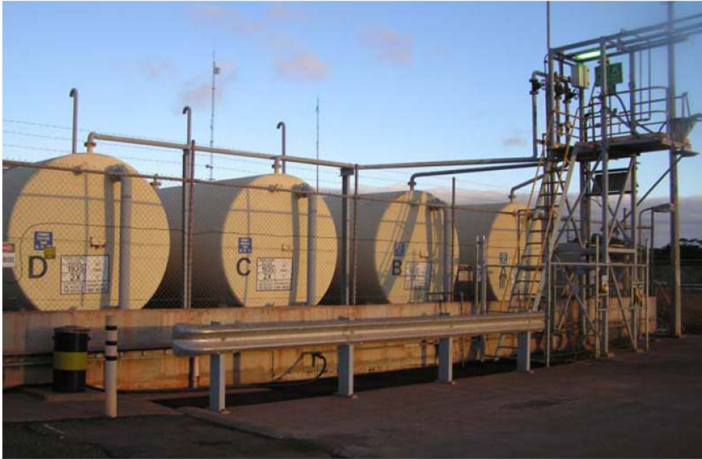
Figure 1.5 Cyanide Storage Bullets at Gidji
